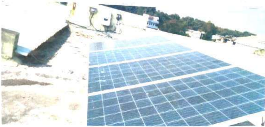
Solar panel on college terrace
